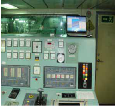
Fig. 4. Control room for main-engine
